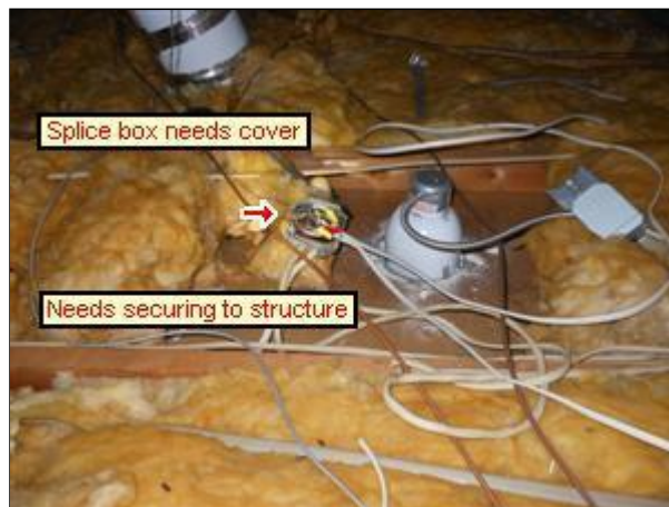
7.2 Picture 3 Splice box needs cover and secured to structure
