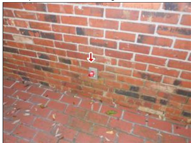
7.3 Picture 2 Receptacle needs GFCI and cover
