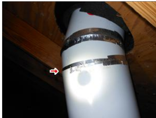
9.4 Picture 1 Joint in pipe needs repaired
