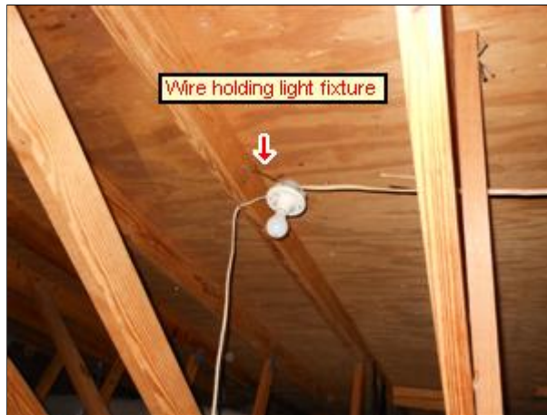
7.2 Picture 4 Light fixture needs securing to structure
