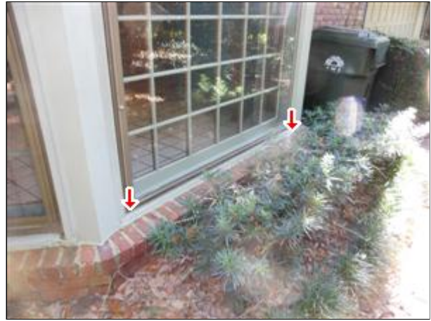
2.0 Picture 2 Water damage at window
