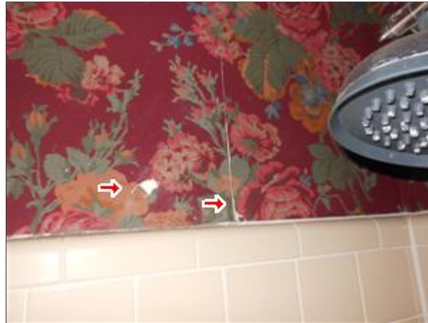
4.1 Picture 1 Wallpaper torn and loose on wall
