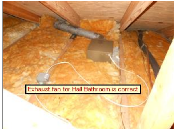
9.2 Picture 2 Exhaust fan terminates at the soffit
