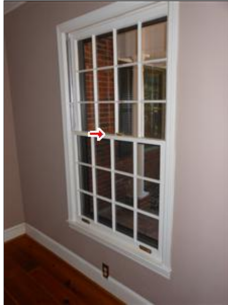
4.5 Picture 1 Latch broken
