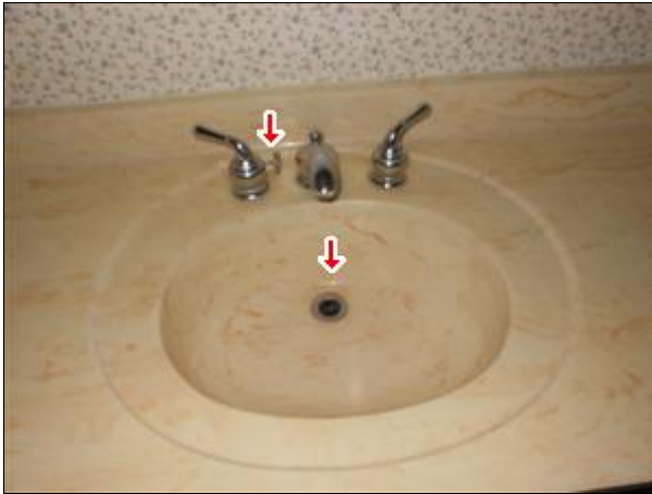
6.1 Picture 1 Stopper removed and doesn't work
