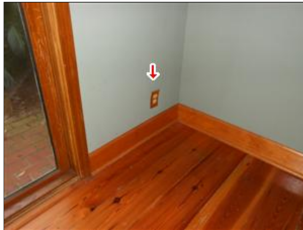
7.2 Picture 2 Receptacle needs repairs
