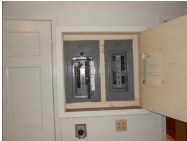
7.1 Picture 1 Federal pacific Panels
