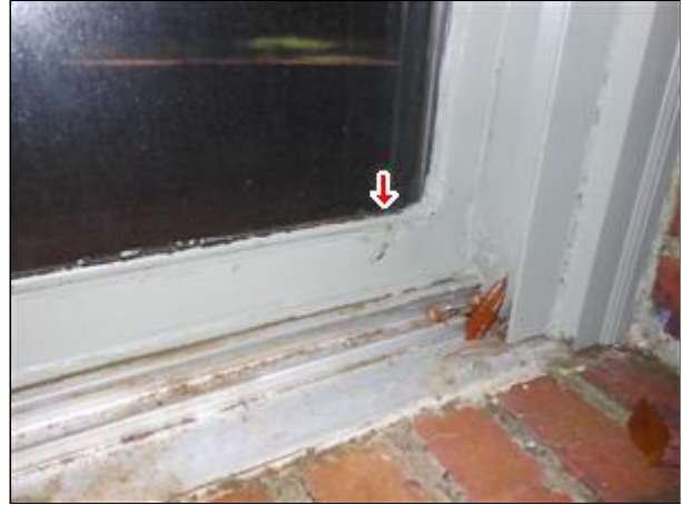
2.1 Picture 3 Water damage at sliding glass door
