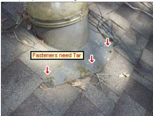
1.2 Picture 1 Fasteners need tar
