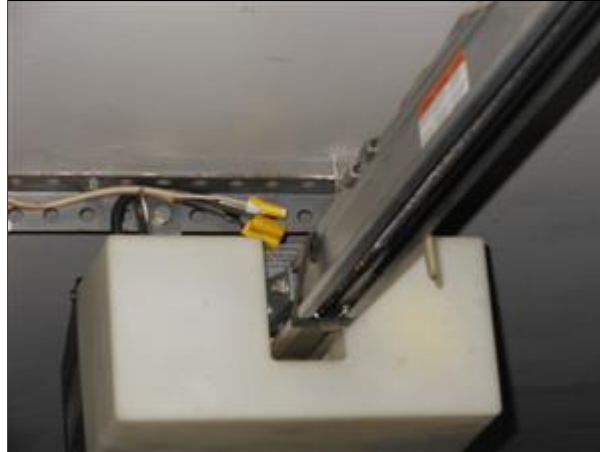
3.5 Picture 1 Garage Door Electrical connection not complete
