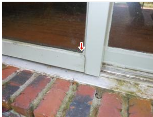
2.1 Picture 4 Water damage at sliding glass door
