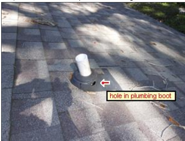
1.2 Picture 4 Hole in Plumbing stack boot
