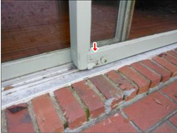
2.1 Picture 2 Wood sliding door damaged
