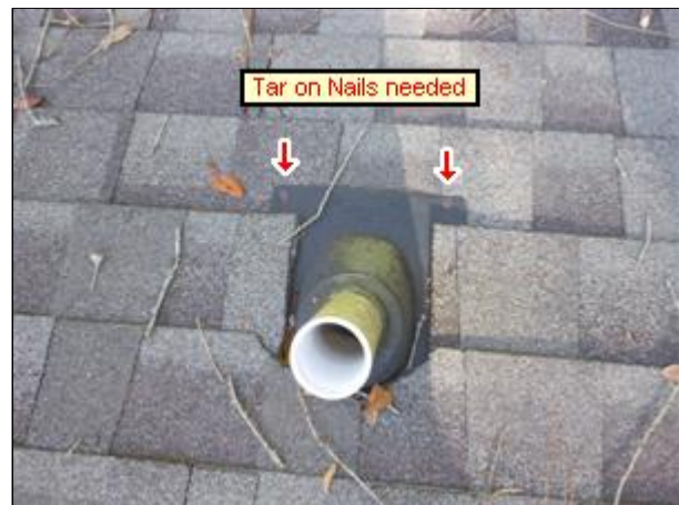
1.2 Picture 2 Fasteners need tar
