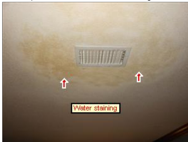
4.0 Picture 1 Water staining on ceiling
