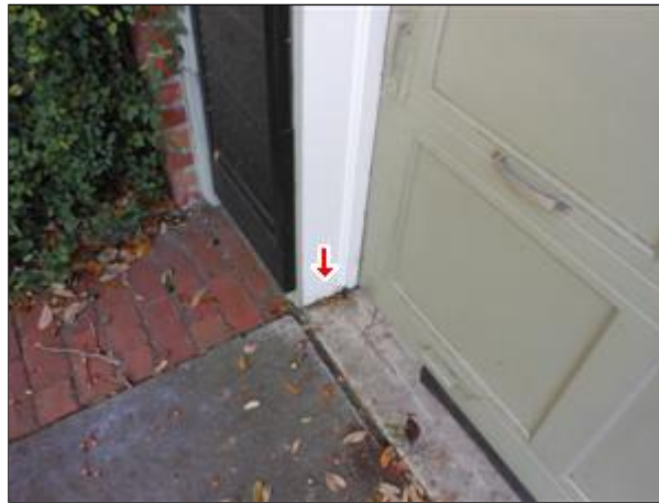
2.0 Picture 3 Water Damage to wood trim
