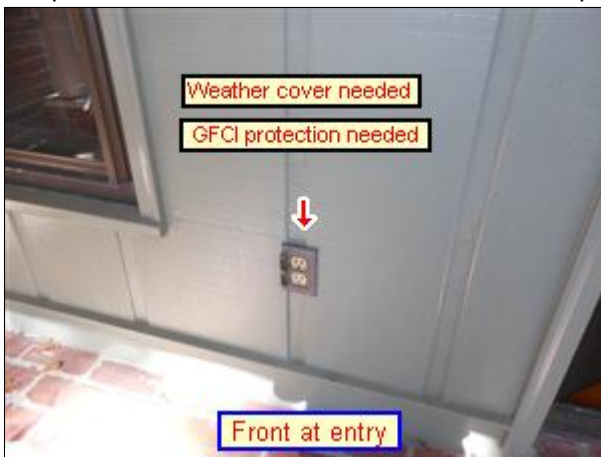
7.3 Picture 1 Receptacle needs GFCI protection and cover
