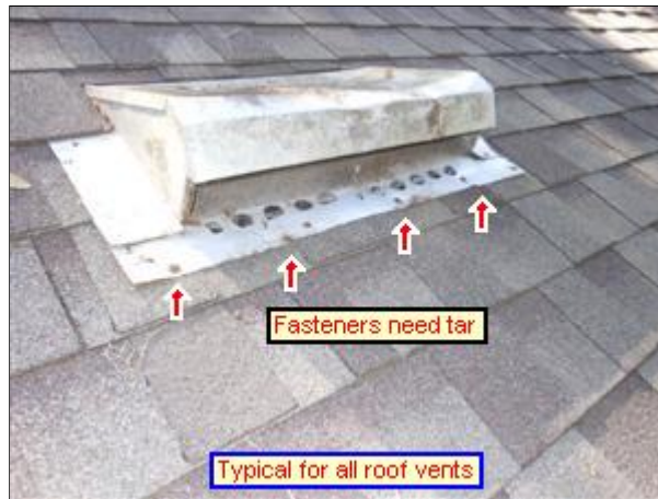
1.2 Picture 3 Fasteners need tar
