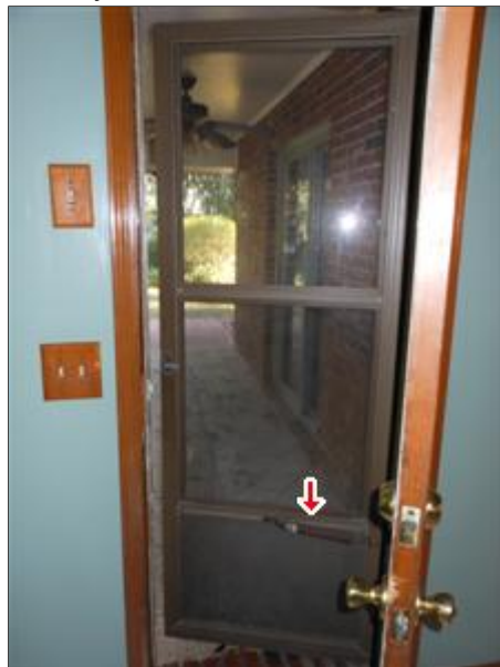
2.1 Picture 1 Broken closer
