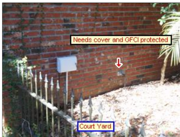
7.3 Picture 3 Receptacle needs GFCI and cover
