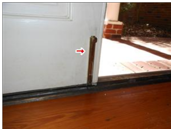
4.4 Picture 1 Door Bolt needs repairs
