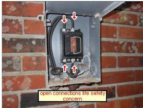
7.2 Picture 1 Electrical disconnect is easily accessible and is a life safety concern.
