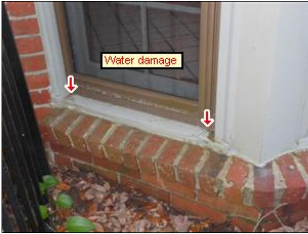
2.0 Picture 1 Water damage at window
