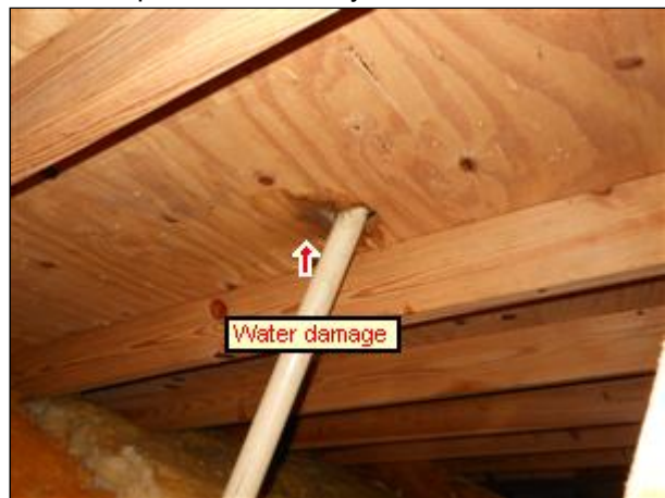
1.2 Picture 5 Water staining on plumbing stack that has the broken boot
