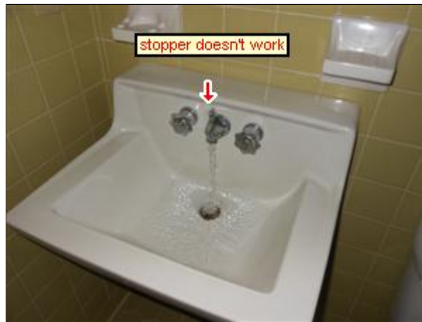
6.1 Picture 3 Stopper doesn't work
