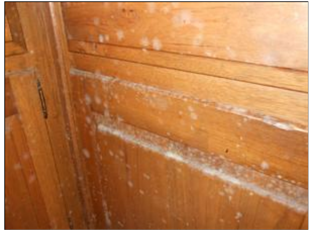
4.3 Picture 2 Mold on cabinets
